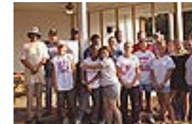
<< River Way work team takes a break while constructing a new porch
